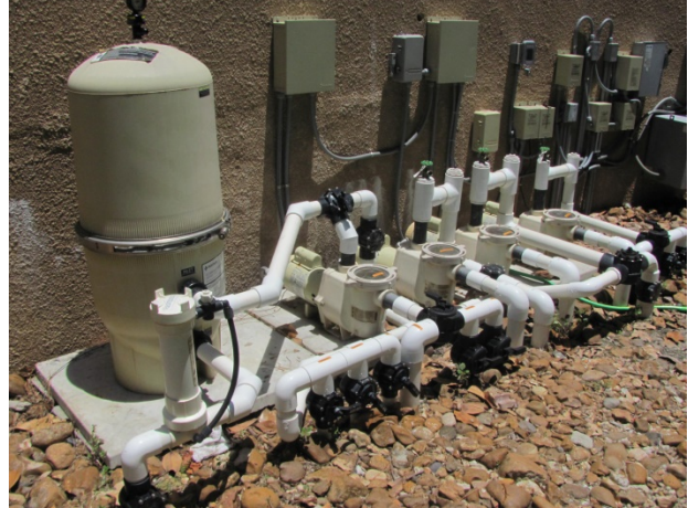
Filter and pumps
