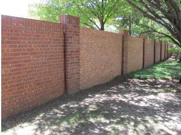
Previous repairs at perimeter wall
