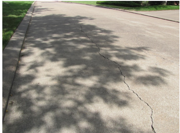
Isolated section with settlement and significant cracks at Noblewood Boulevard
