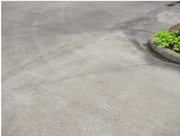
Cracks and standing water evident at Royal Oaks Club Drive
