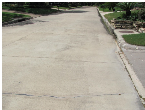
Cracks and standing water along curb at Antibes Lane
