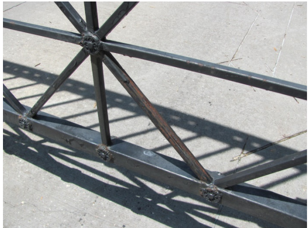
Rust at steel gate
