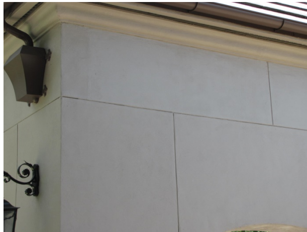
Stucco discoloration at main guard house
