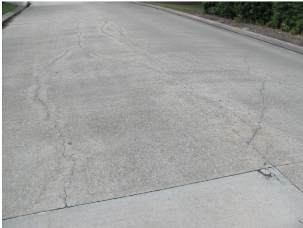
Various cracks and deterioration at Gallant Ridge Lane
