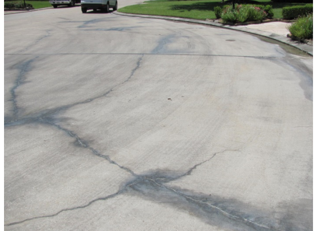
Various cracks and standing water along curb at Versailles Lakes Lane
