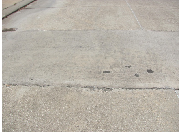
Concrete spalls and deterioration at Tudor Manor
