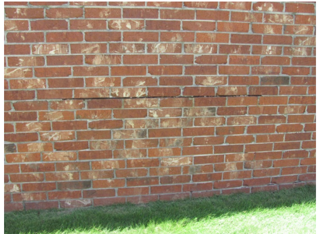
Loose mortar evident and rust at steel support
