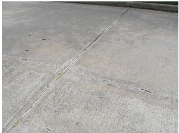
Cracks and deterioration along joint at Legend Manor Drive
