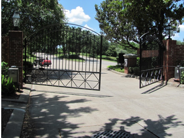
Bi-parting gate and operators
